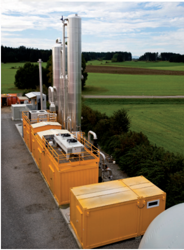
The methane upgrading plant in Altenstadt/Baden-Wuerttemberg which is fully operated with biogenic waste. photos: erdgas schwaben gmbh
