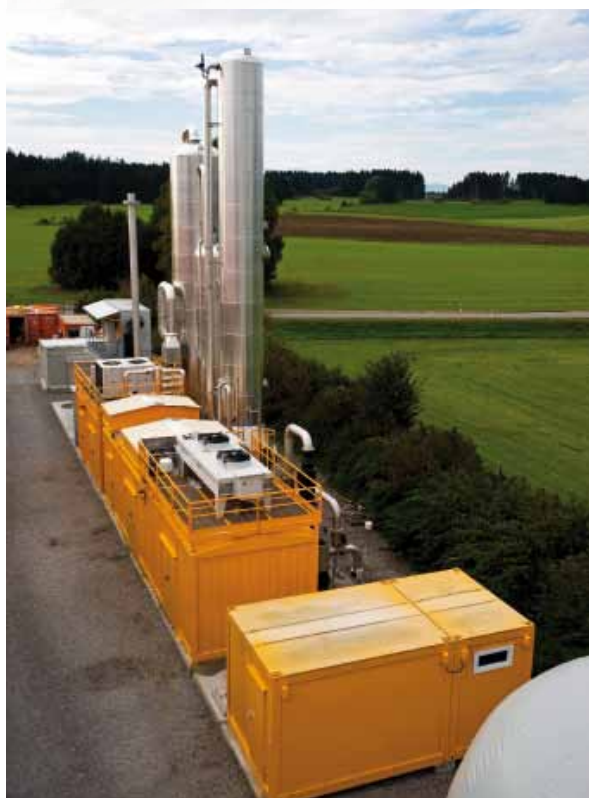
The methane upgrading plant in Altenstadt/Baden-Wurtemberg which is fully operated with biogenic waste. photos: erdgas schwaben gmbh
