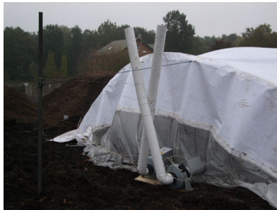
Ambient air supplied to the wind tunnel with two separately installed fans and supply air ducts (front view of the wind tunnel)
