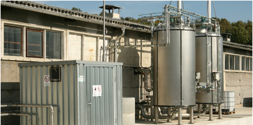
Figure 7.3-3: Pilot biogas plant Fraunhofer IKTS
