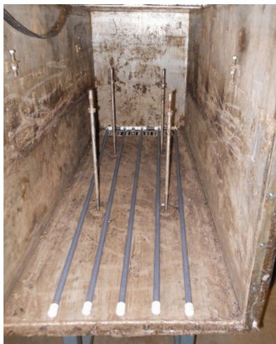
Figure 8.7-4: Aeration header in the base of the dry digester converted for use as an aeration bunker, the vertical rods for the substrate compression system are also visible (Source: InnoTech)
