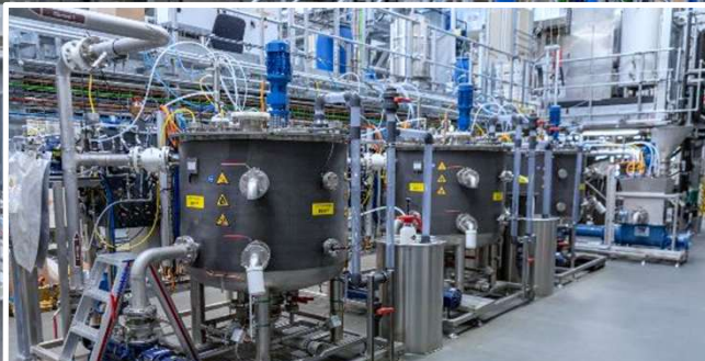
Anaerobic fermentation| Line 1
